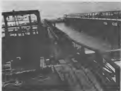
At left is the old wooden baffle at the Secondary Separator and concrete wall, at right is the new baffle. Na robex ta e muraya bieuw di madera na Separator Secundario y e muraya nobo di concret y staal, na...
